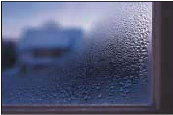
Condensation on the inside of a windowpane.
